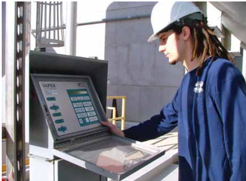
Kyle Curtis of the HRSD at the control panel of the Vapex continuous gas analyzer.
