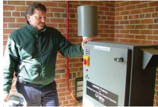
The sanitation district's environmental scientist Mark Feltner with the Vapex O-Mega odor-control system.
