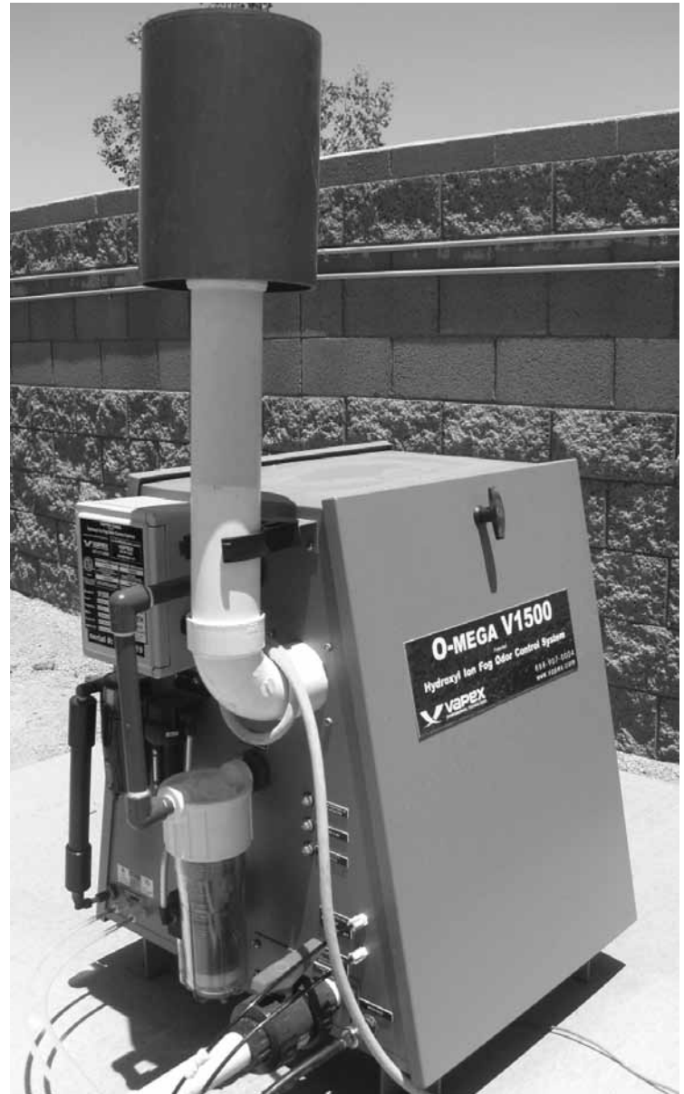
A Vapex O-Mega V-1500 ion-fogging system is helping control odors at a 2 mgd lift station in Maricopa, AZ.
