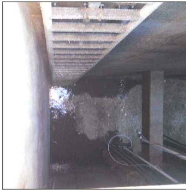
Figure 6: May 20, 2011 – 8 days after cleaning with Vapex treatment
